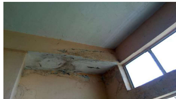
Fig.2.1.5 Defect occurred due to Dampness
