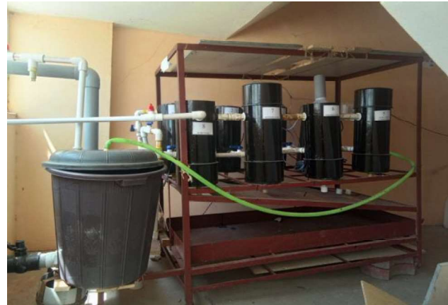
Figure 1. Compact waste water treatment unit
